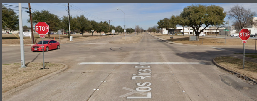
Figure 4. Northbound on Los Rios Boulevard at Merriman Drive- The City of Plano Transportation Division identified that pedestrian ramps were present at all four corners of the intersection, but crosswalk pavement markings were missing at all four approaches.
