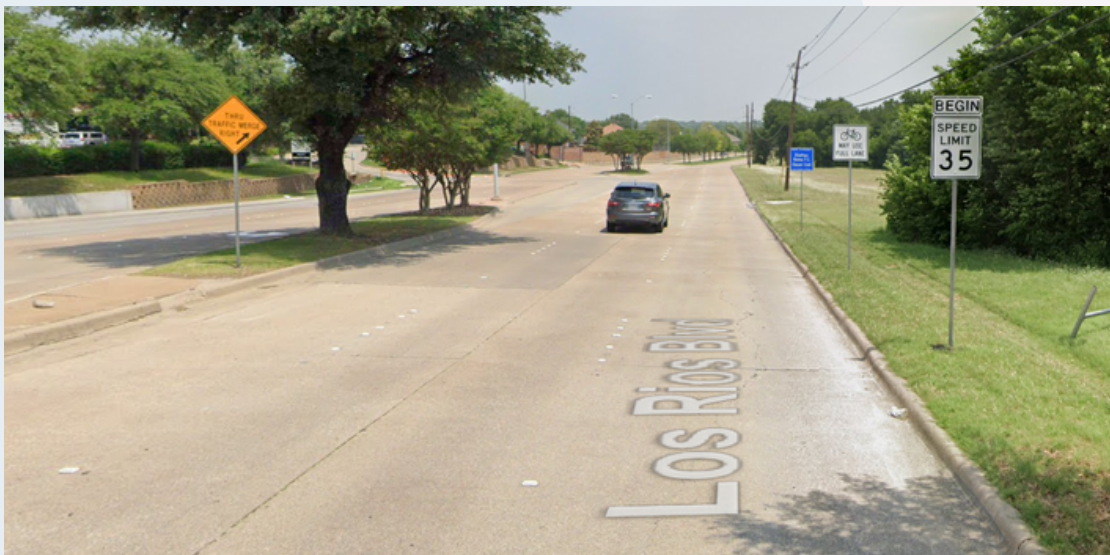
Figure 7. Northbound Los Rios Boulevard at 14th Street- The City of Plano Transportation Division identified insufficient and incorrect use of signs and pavement markings in order for drivers to taper and merge properly for the inside lane drop traveling northbound on Los Rios Boulevard north of 14th Street.
