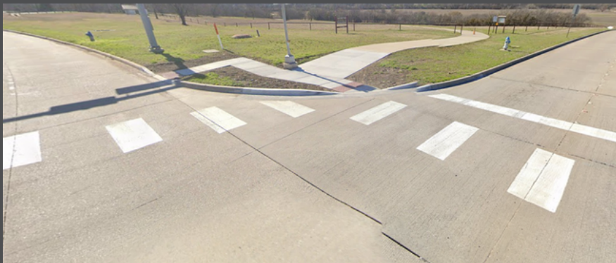
Figure 3. Los Rios Boulevard and Parker Road- The City of Plano Transportation Division identified crosswalk pavement markings that were not aligned with the pedestrian ramp in the northwest corner.
